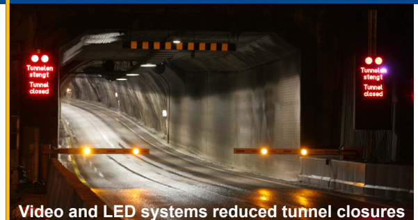
Video and LED systems reduced tunnel closures
